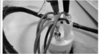
Picture F13-2: 220VAC control on U outlet ends of the noise filter
